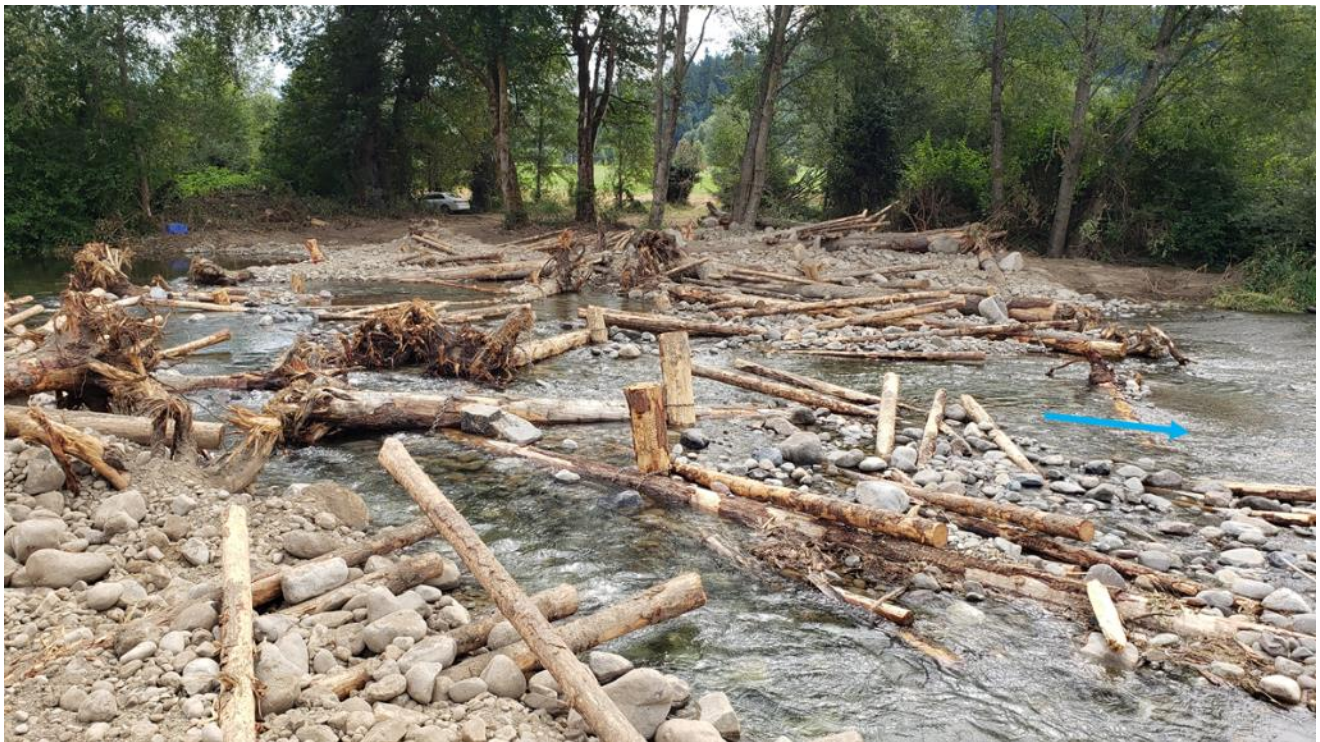
Figure 27. Channel-Spanning Engineered Logjam in South Prairie Creek, Pierce County, Washington Immediately following Construction
